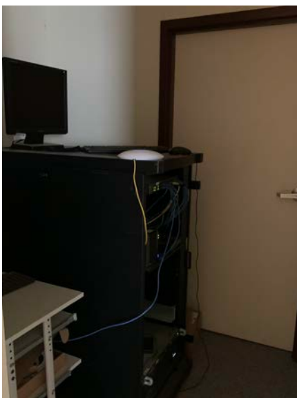
Small Server room, no ventilation
