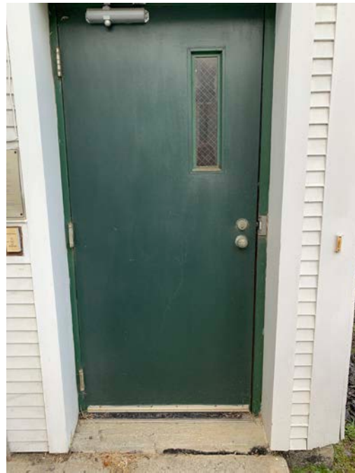
Handicapped elevator door. Note the cement is not even with the sidewalk, making it impossible to independently lift a wheelchair into the elevator. Door is heavy and does not open automatically. There is no official handicapped parking.
